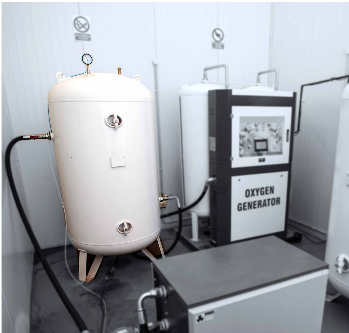
Figure 9. Compressed air storage tank
