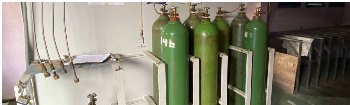
Figure 17. Cylinder filling station
