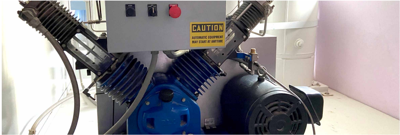
Figure 16. Booster compressor for cylinder filling.
