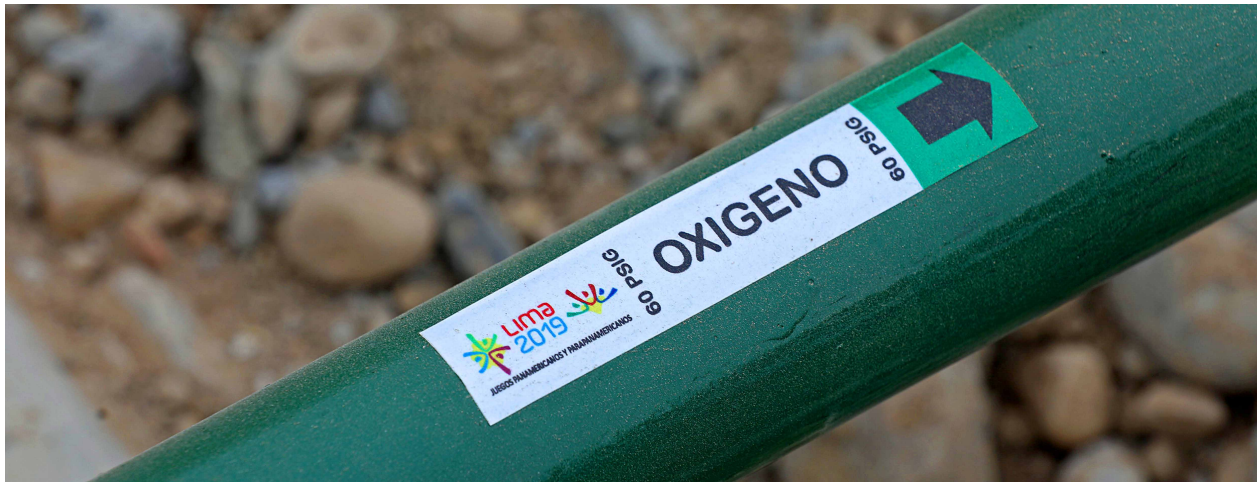
Figure 12. Medical gas supply system
