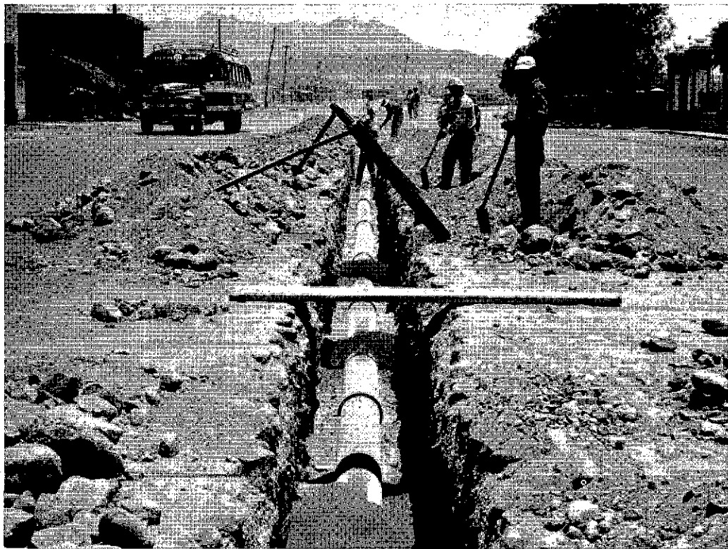
POTABLE WATER COMES TO URBAN CONSUMERS—WORKMEN LAYING A SECTION OF 10-INCH, ASBESTOS-CEMENT WATER MAIN IN AREQUIPA, PERU.
