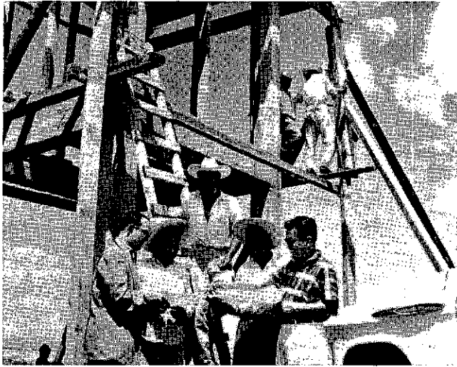
Construction of water tank being accomplished by villagers, under the guidance of an engineer, Tavera, Guanajuato, Mexico.
