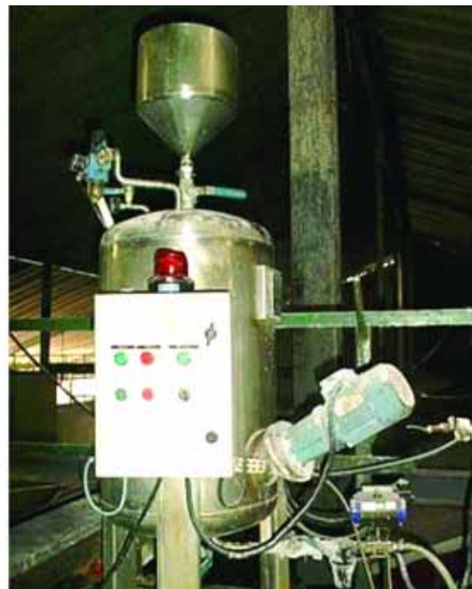
FIGURE 5.9 Wet method equipment: dosing solution mixer and “egg” type pump driven by compressed air.
