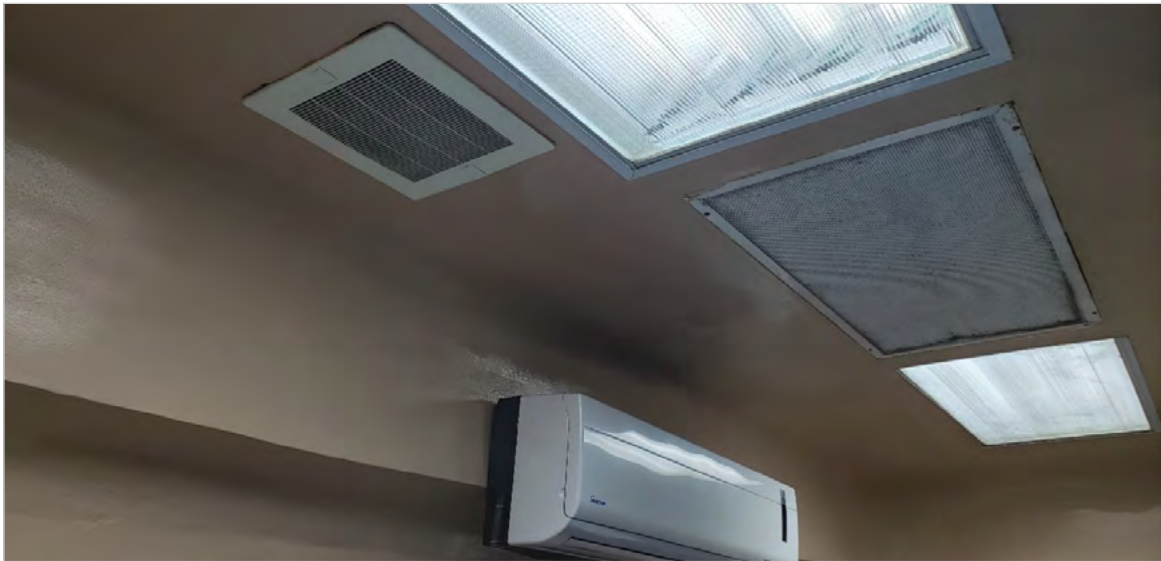
Figure 7. Mini split systems in operating rooms are not recommended
