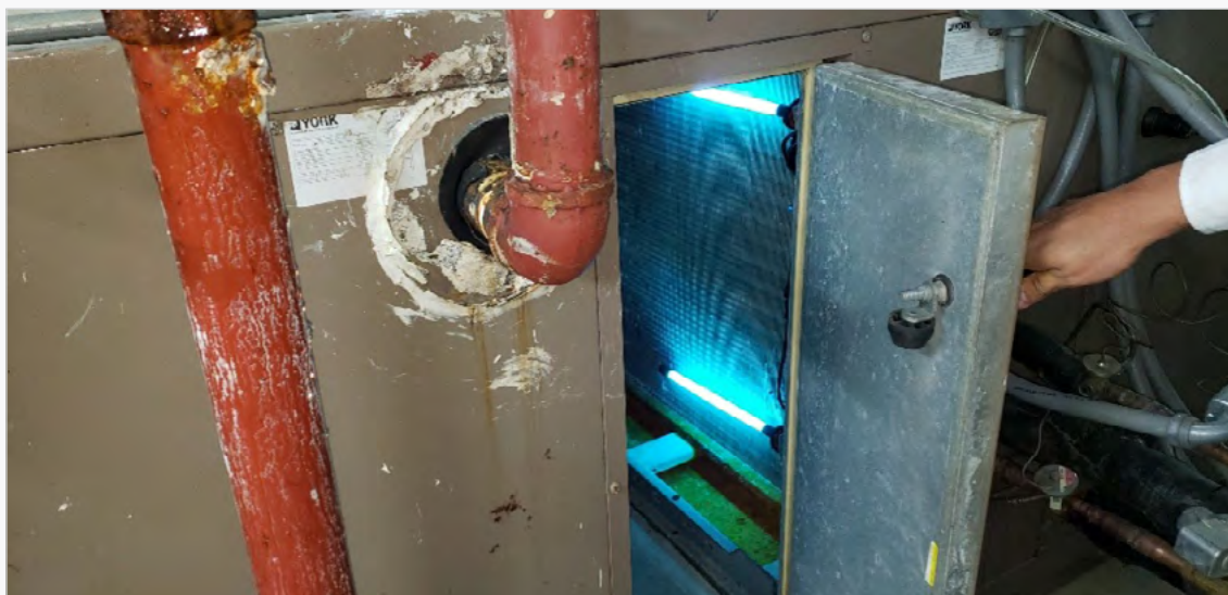
Figure 9. UVGI lamps installed upstream of the cooling coil
