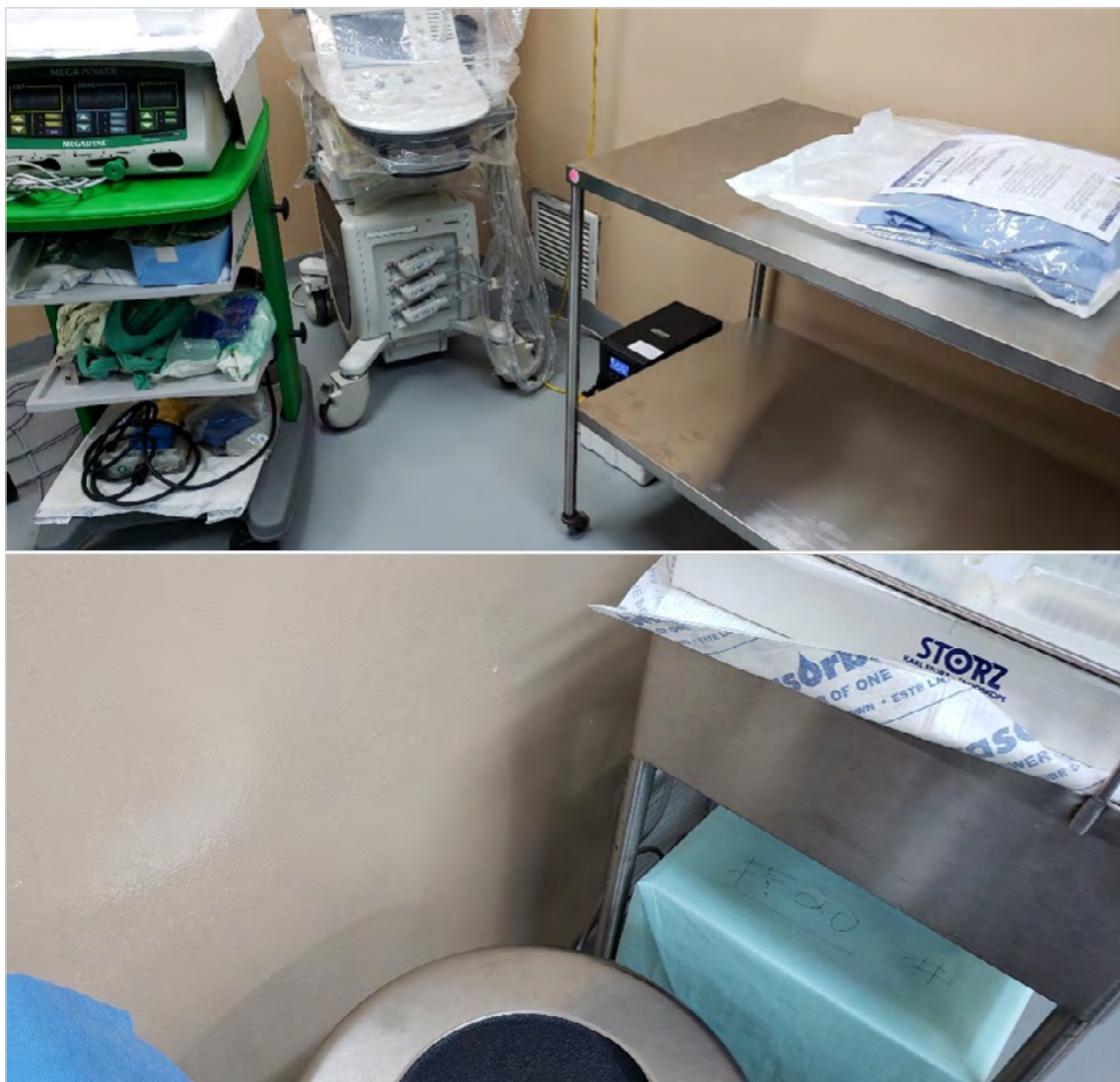
Figure 8. Return grilles should be free of obstructions
