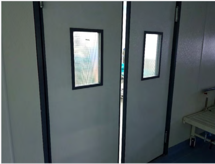
Figure 4. Doors to an operating room that do not seal properly
