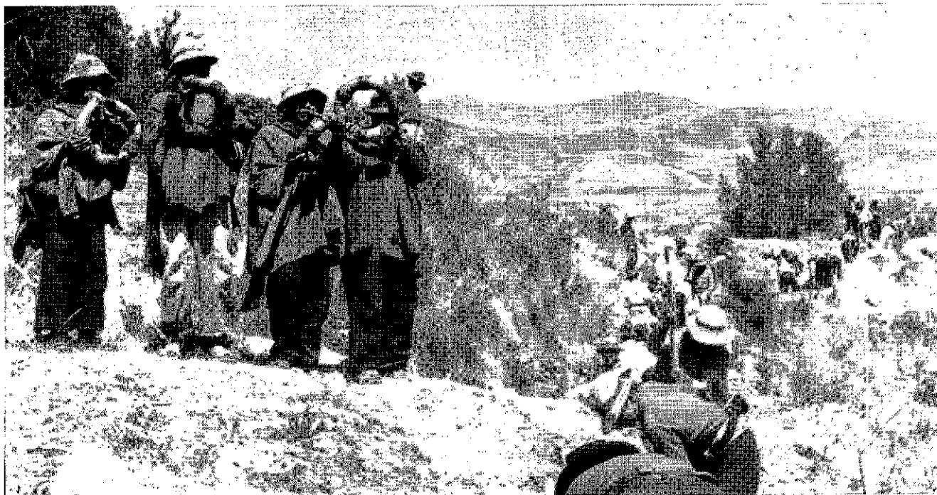
Villagers in the Andean highlands of Peru join in the construction work on a rural water supply system.
