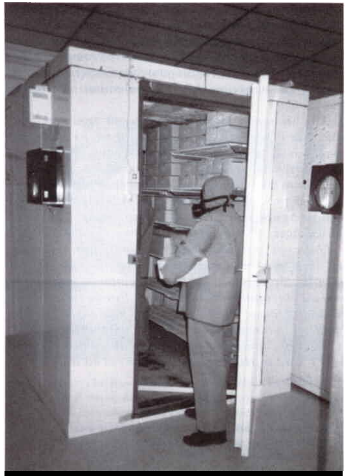
Proper vaccine storage and cold room management at the central level are absolutely essential to insure that potent vaccines reach the clinics where they will be used in immunization programs. (Photo: Fernando Laender/PAHO)
