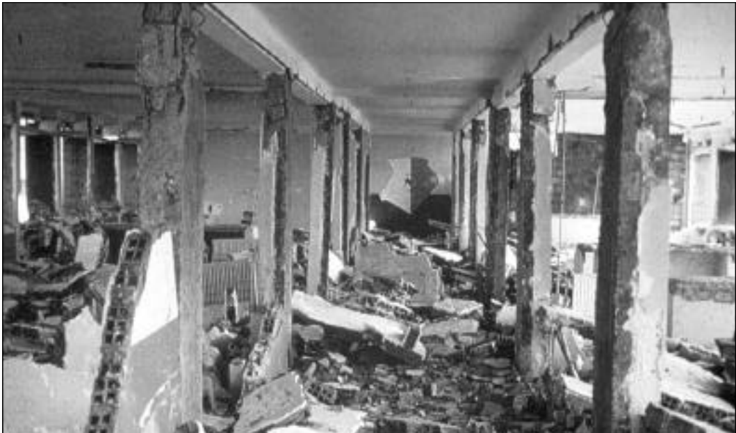
Photograph 24. Walls destroyed due to flexibility of the structure
