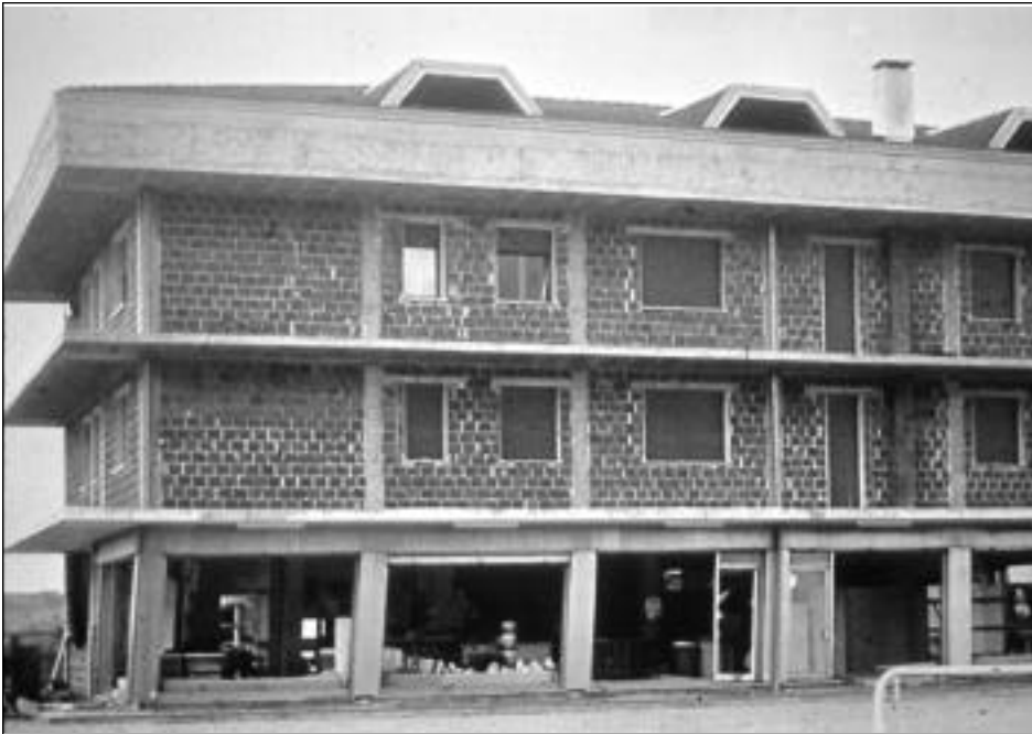
Photograph 9. Failure on ground floor due to soft story.
