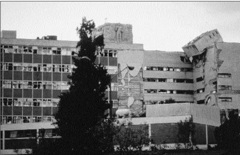
Photograph 8. Concentrations of mass, such as water tanks placed on the roof of a hospital, can cause severe damage in earthquakes.
